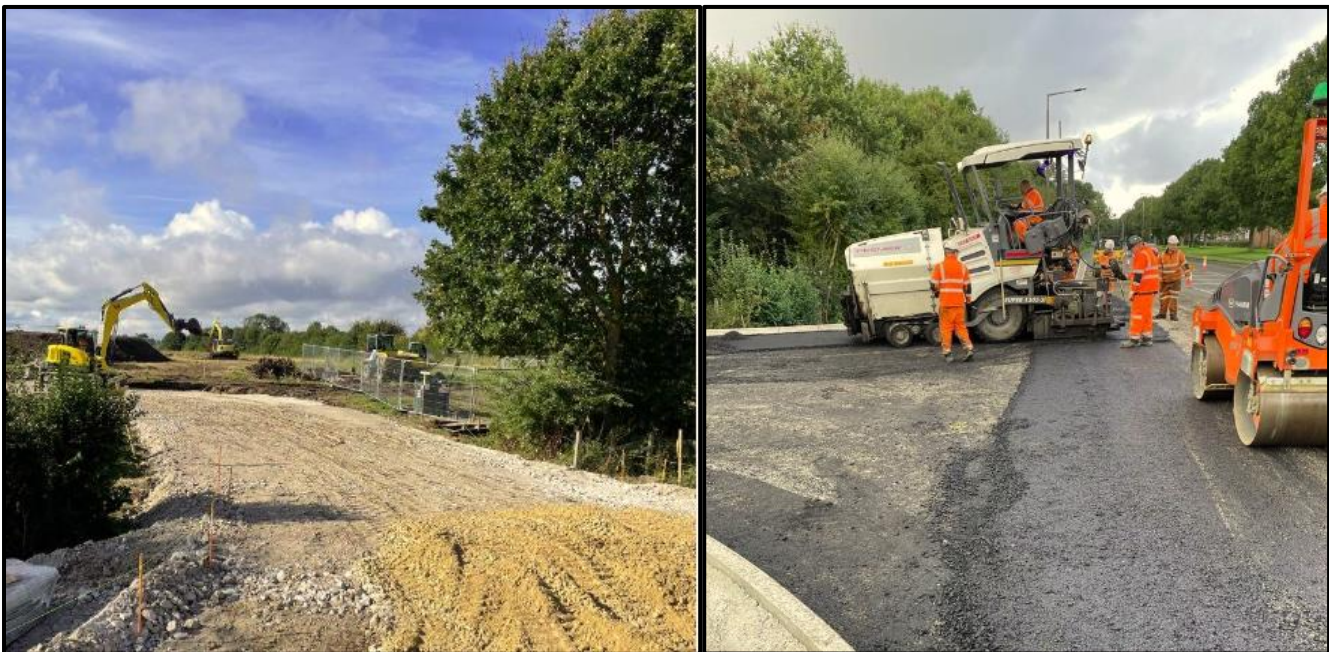
Surfacing work in the cornfield and tarmacking the compound entrance off Shipton Road
